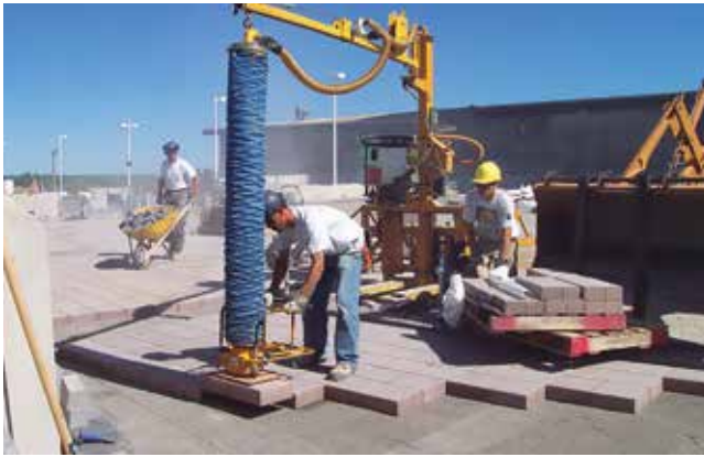
Figure 11. Self-contained vacuum lifter with boom
