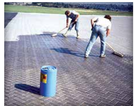
Figure 10. Urethane is applied with squeegees to stabilize joint sand between pavers on aircraft pavement.
