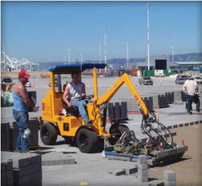
Figure 15. Spacing of cubes at the laying face is determined by how much area will be covered by each, as well as by the clearance required by the machine clamp. Orientation of the cubes follows the direction of paving.
