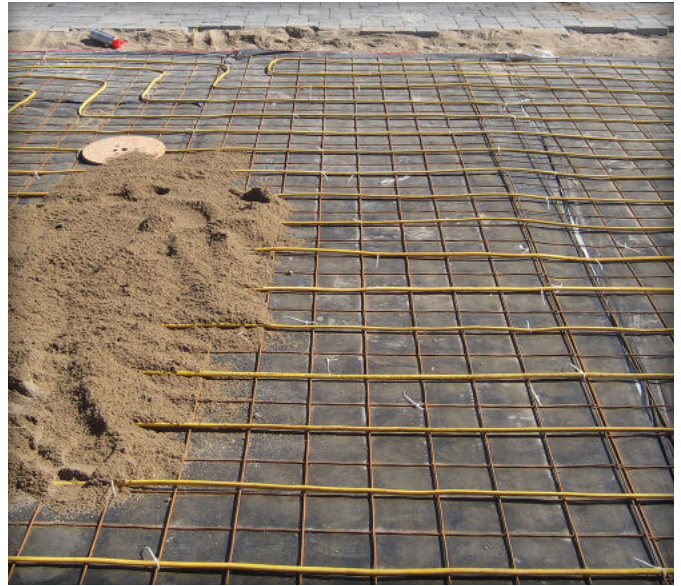
Figure 7. Spreading and screeding bedding sand must be done without moving or damaging pipes or wires for melting snow.
