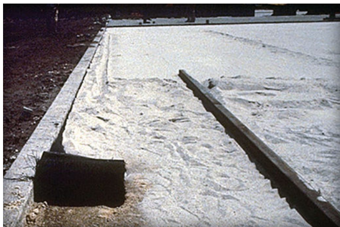
Figure 7. Woven geotextile used to contain bedding sand from migrating laterally. Visit www.masonryandhardscapes.org for detail drawings.
