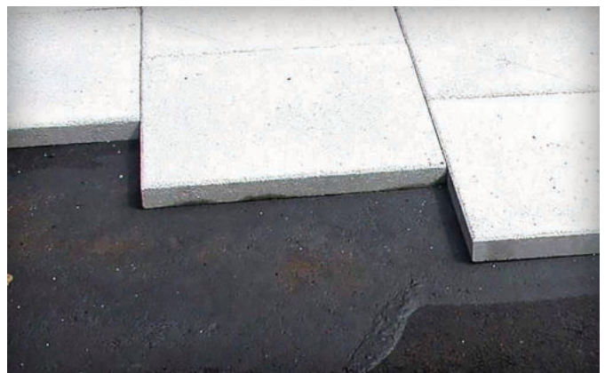
Figure 8. Sidewalk application illustrating the neoprene adhesive on an asphalt bedding layer under paving slabs
