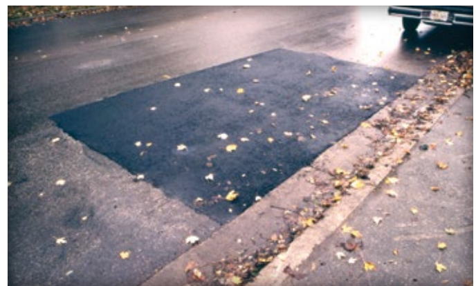
Figure 7. Pavement damage from settlement and shrinkage of cold patch asphalt.
