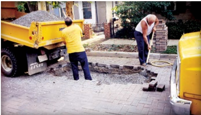
Figure 2. Removal of concrete pavers for a gas line repair in Dayton, Ohio.
